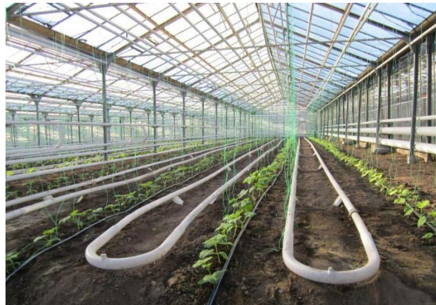
Picture 1 The heating system with smooth tubes
