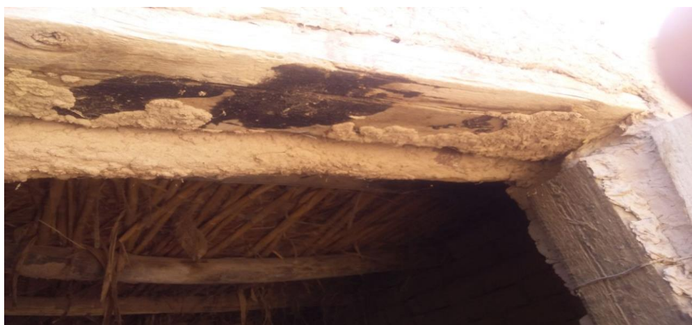
Figure 2: Termite damage to houses in Denau district
