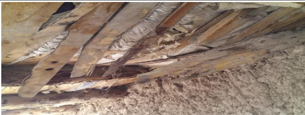
Figure 1: Houses in "Khalkabad" mahalla of Termez district termite damage
