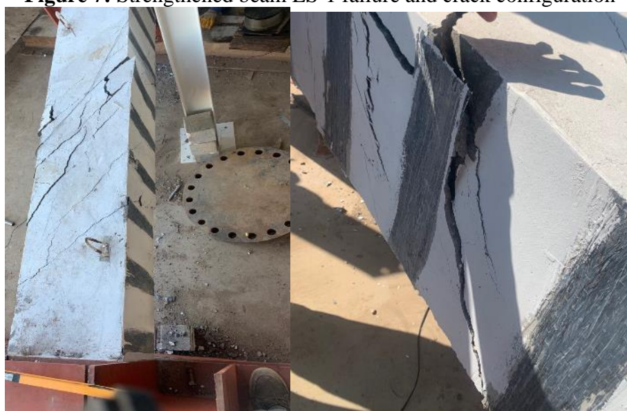
Figure 8: Strengthened beam ES-2 failure and crack configuration.
