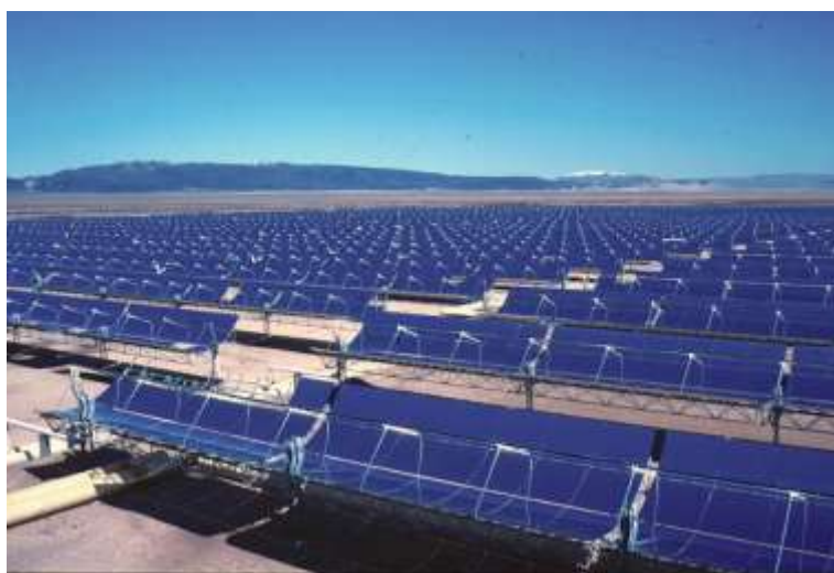
Fig. 1. Modular installations of solar power station Solar Energy Generating Systems, California (USA).
