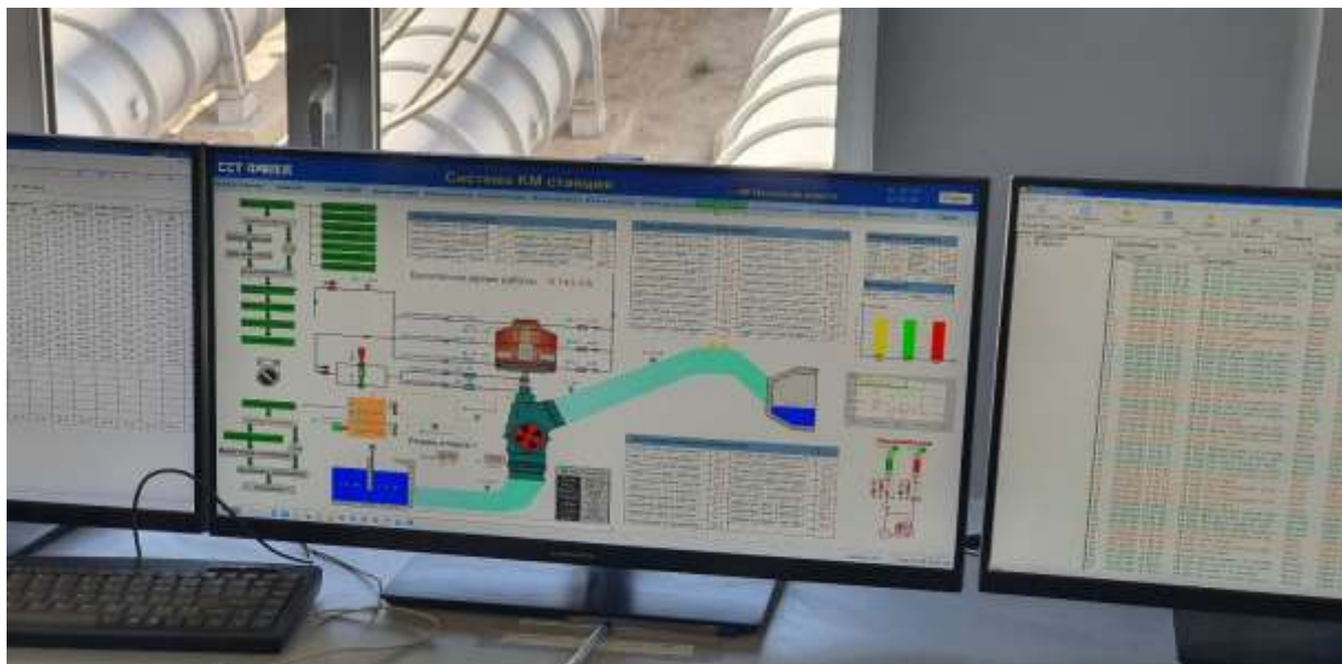
Figure 2. Pump station control room.
