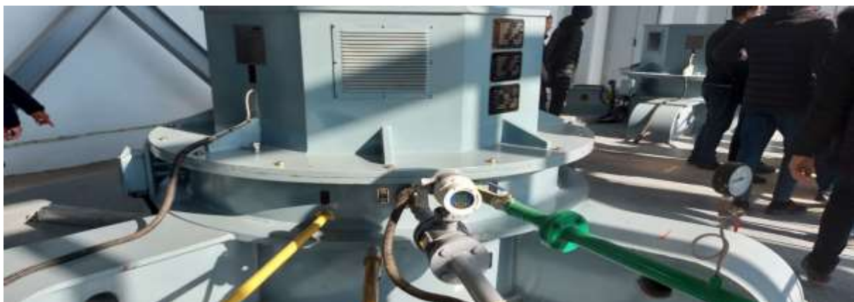
Figure 1. Pump units installed at the foundry pumping station.
