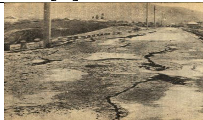
Fig. 7. Damage to the dam of the Chiryurt hydroelectric power station during the Dagestan earthquake on 05/14/1976 [7]
