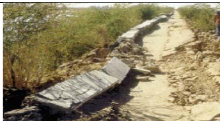
Fig.8. Longitudinal cracks on the upstream face of the Feitigadh Dam (India), caused by the Bhuj earthquake on January 26, 2001[8].
